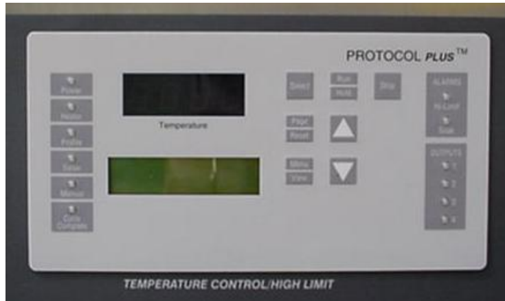
Protocol Plus Controller on upper portion of control panel
