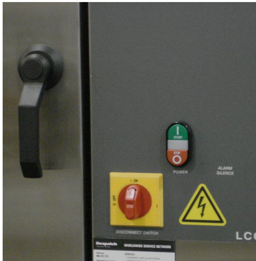
Lower Portion of Control Panel
