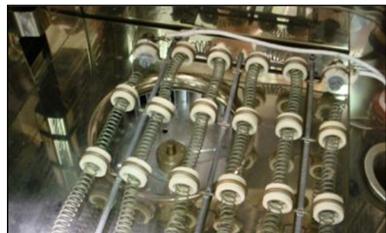
Figure 10. Heater Panel and Inlet Cone.
