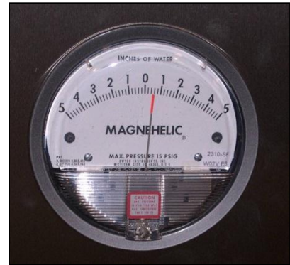
Figure 4. Magnehelic Pressure Gauge Measures Pressure in front of the HEPA filter.
