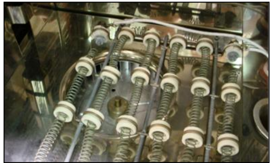
Figure 11. Heater Panel and Inlet Cone.
